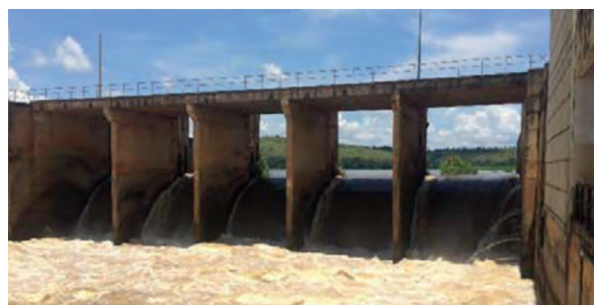
Mobaye dam and hydroelectric power plant – Democratic Republic of Congo
